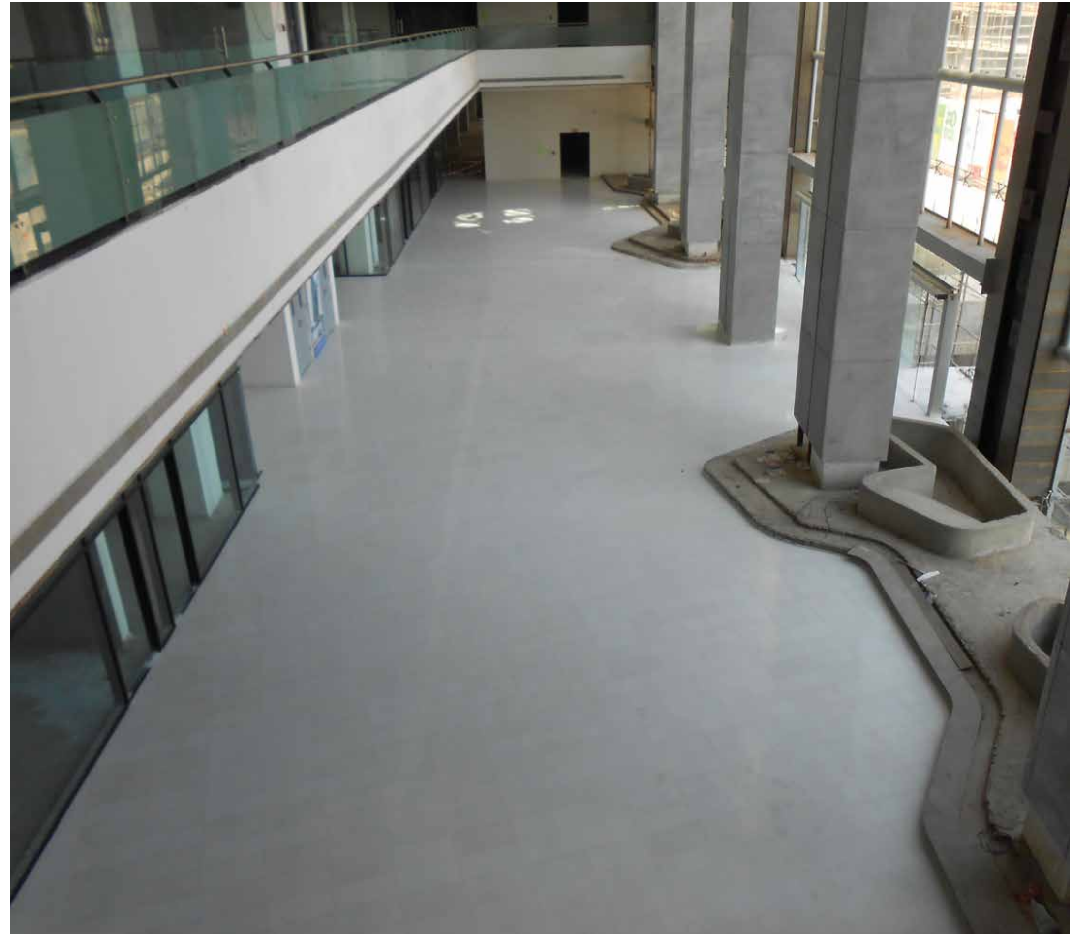
Cast in Situ Terrazzo in Grey and White colours at Tata Consultancy Services offices, Pune.
