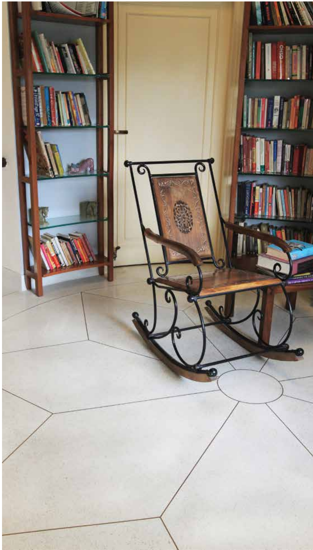
Cast in situ Terrazzo floor done using Brass strips and Cream Italian chips on White base at a private farmhouse in Silver Oak Farms, New Delhi. Interiors: Nikhil Segel. Photographer: Shipra Shrivatava.
